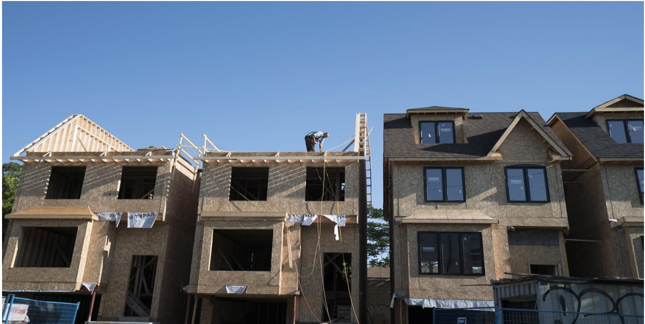
Houses are shown under construction in Toronto on June 26, 2015. THE CANADIAN PRESS/Graeme Roy
