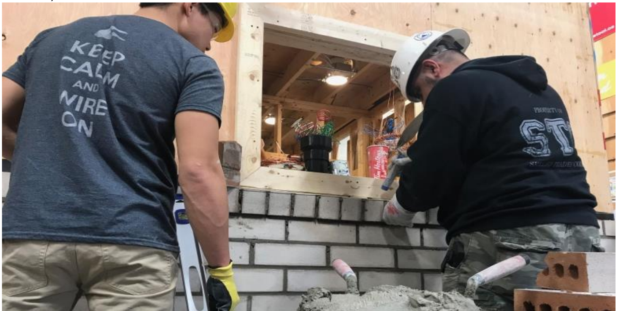
Jimmy Wu and instructor Paul George work together on a brick wall, focusing on the window detailing. (Madeleine Villa/CBC)
