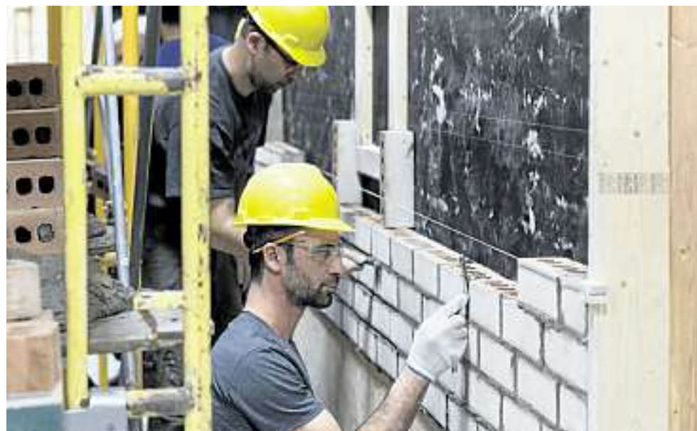
Salah Dib and Dabbah Dib are two of the 10 students learning to build a brick wall in the bricklayers' lab space at the Skilled Trades College of Canada in Vaughan, Ont.
