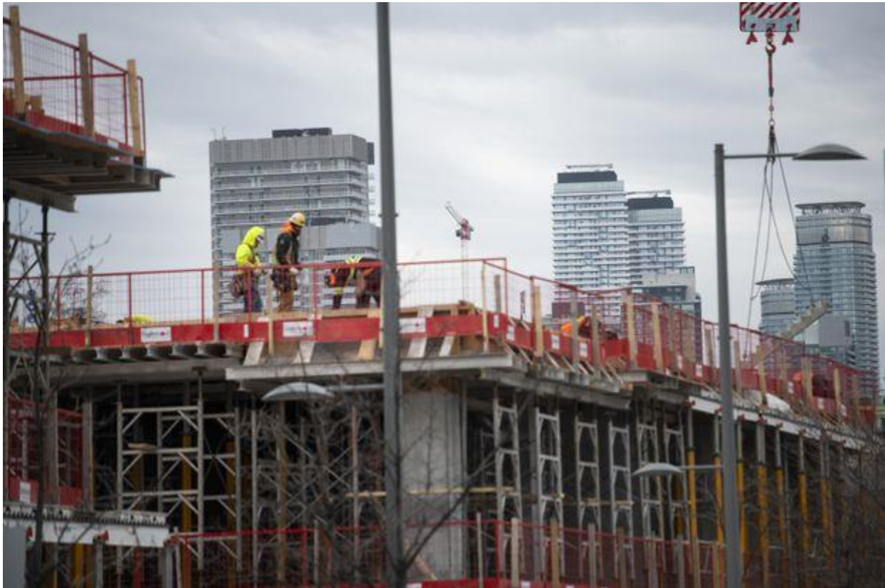
Workers at a condominium construction site near the Distillery District in Toronto on Mar. 16, 2021. Fred Lum/the Globe and Mail
