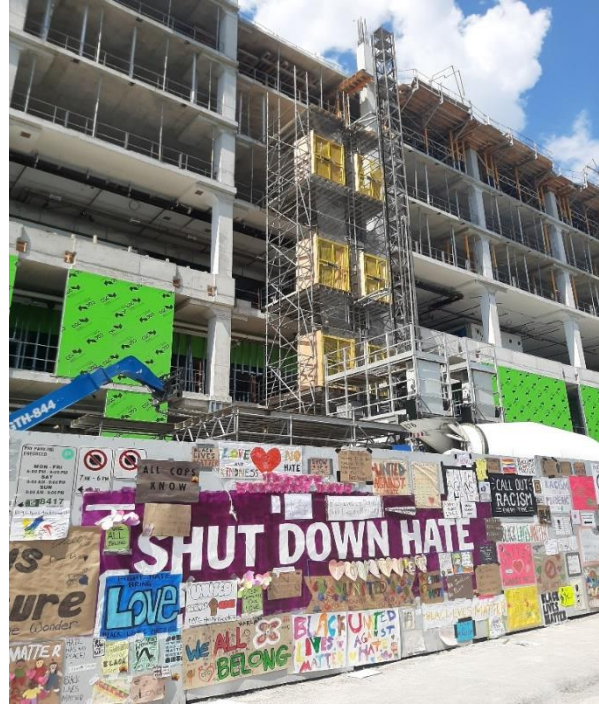
COURTESY OF CARPENTERS' DISTRICT COUNCIL OF ONTARIO — Posters surround a large message that says "Shut Down Hate" at the Michael Garron Hospital construction site. This comes after a noose was found by workers at the site on June 10.
