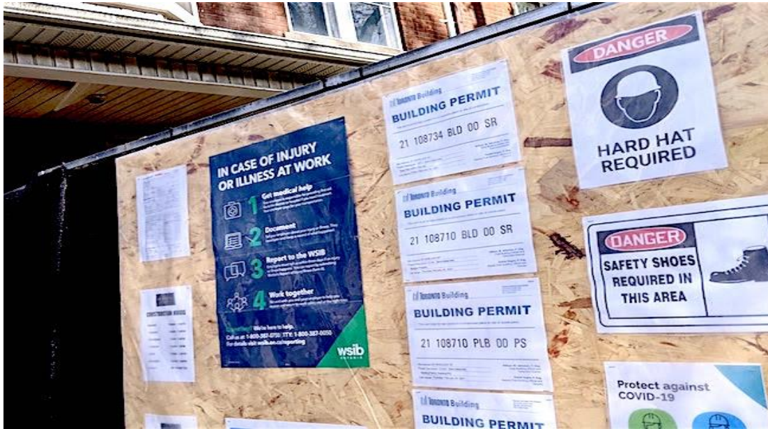
Building permits outside a residential renovation project in Toronto. Advocates say digitization could streamline the permitting process in Ontario and beyond
