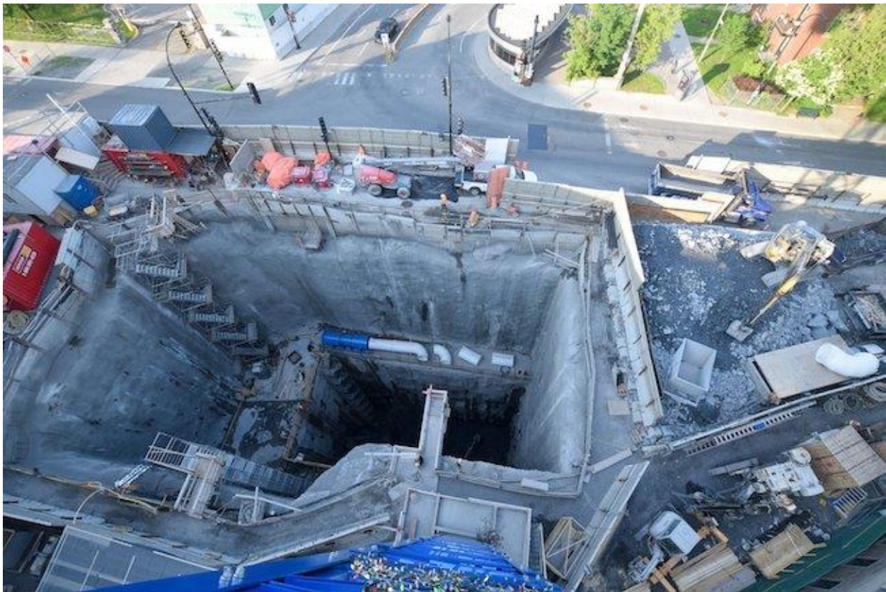
Station construction in Montreal for the city’s new light rail network. PHOTO: REM
